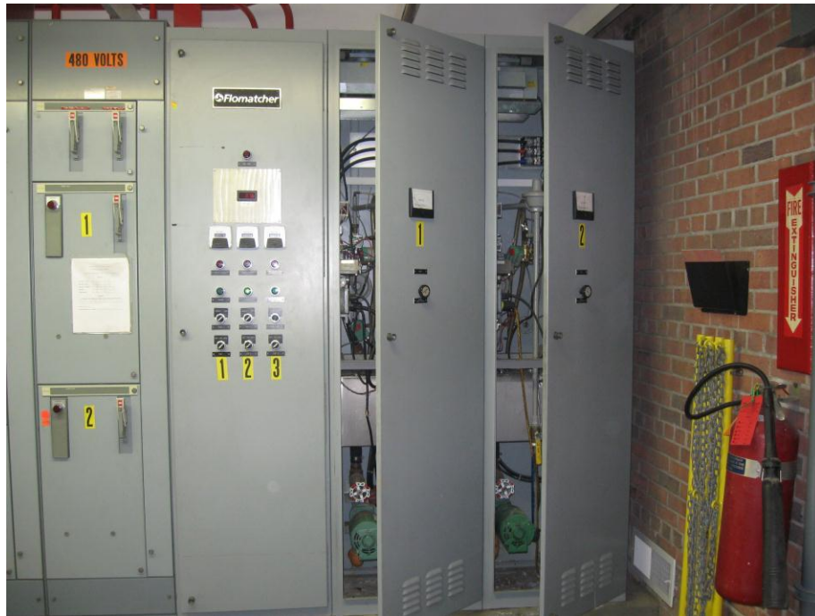
Figure 101-3. Arctic Avenue Pump Controllers
