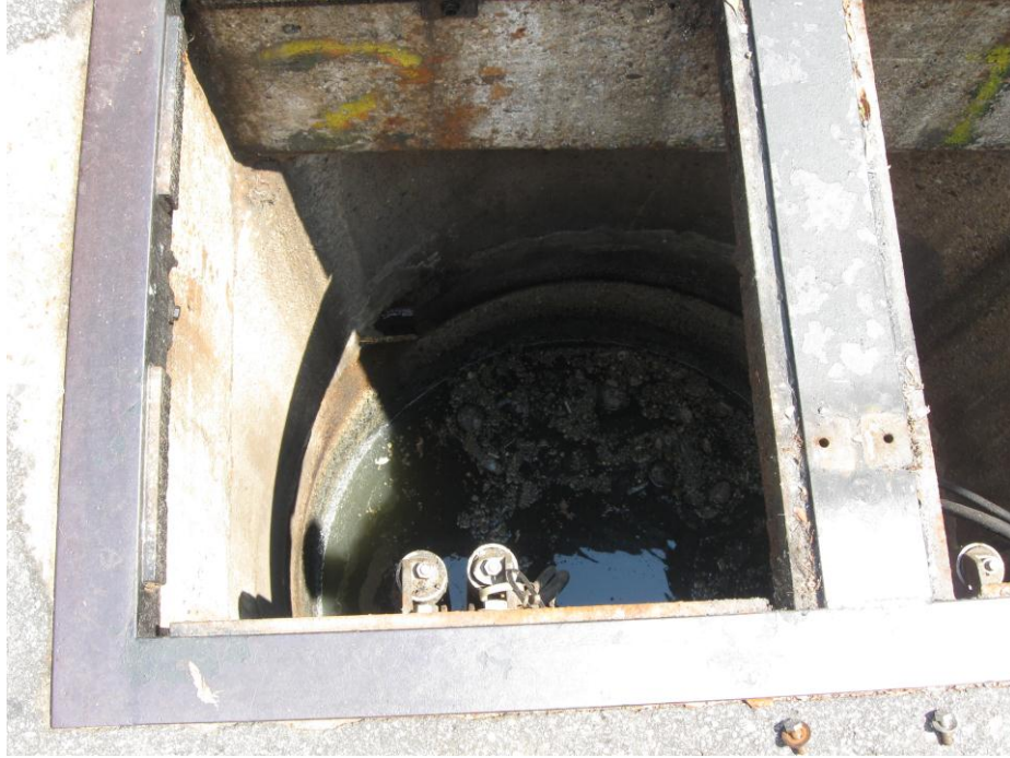
Figure 148-3. Ingleside Rd Wet Well.
