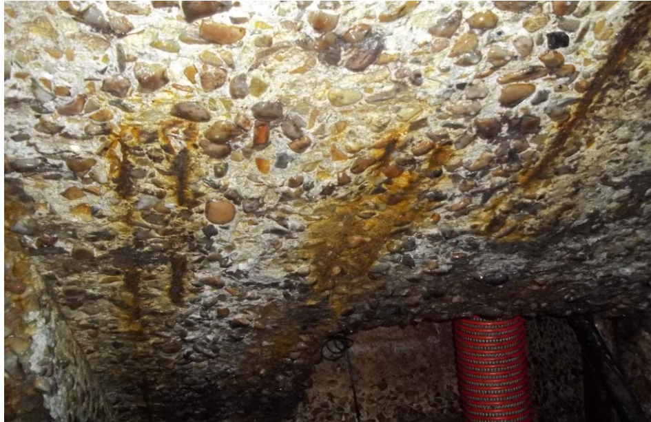
Figure 132-3. Willoughby Ave Wet well
