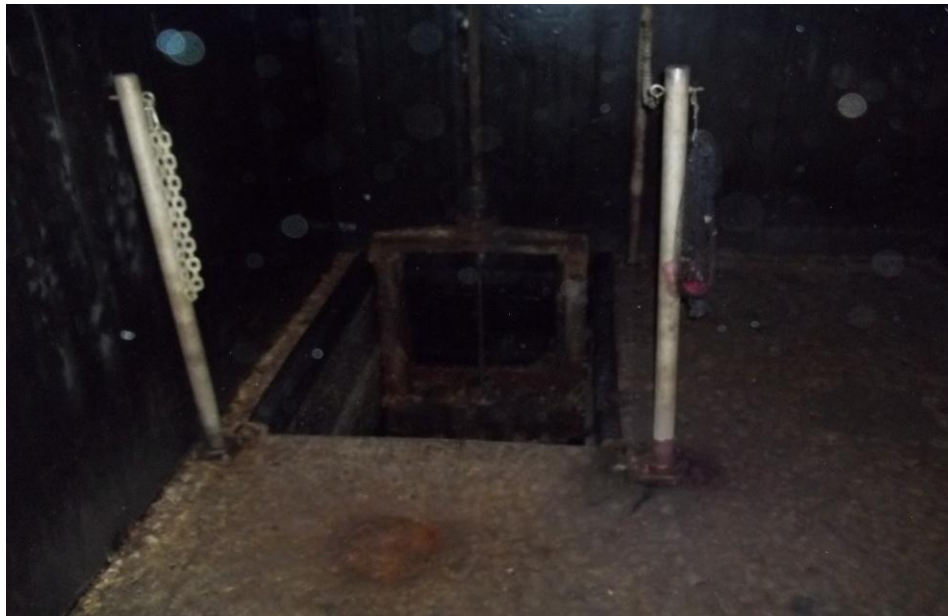
Figure 115-4. Newtown Rd Wet Well
