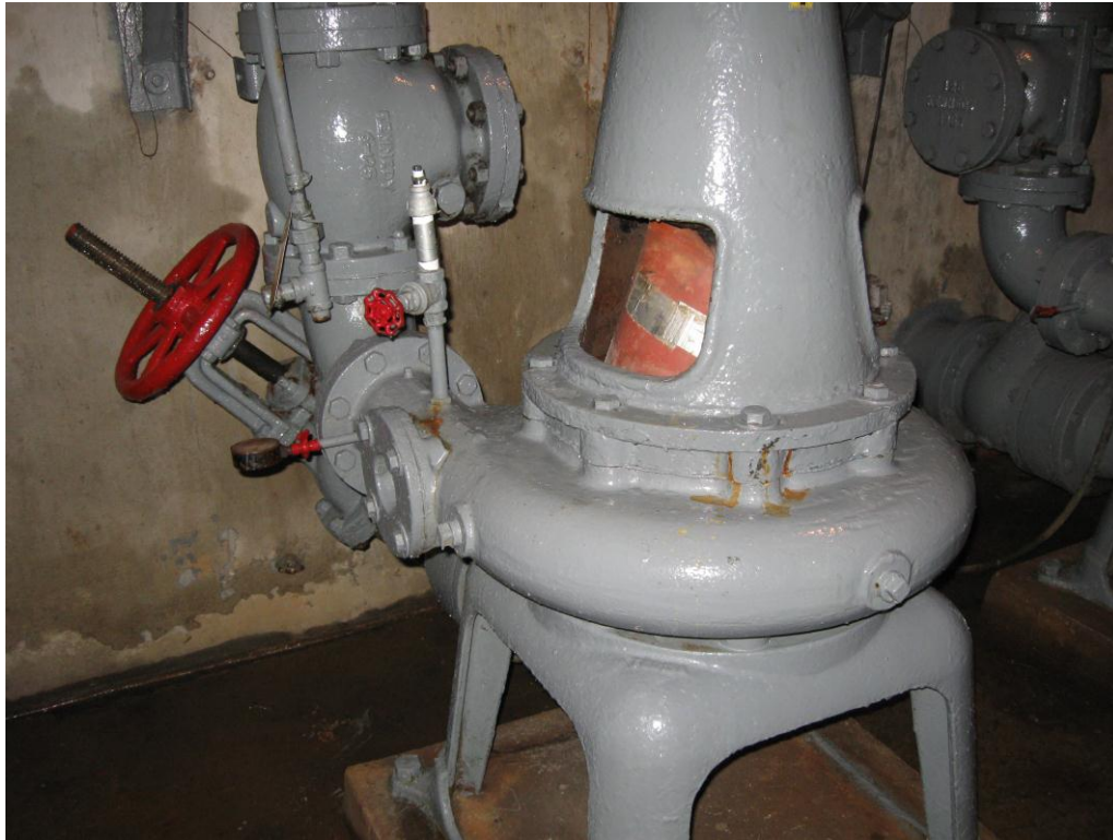
Figure 106-3. City Park Pump Room
