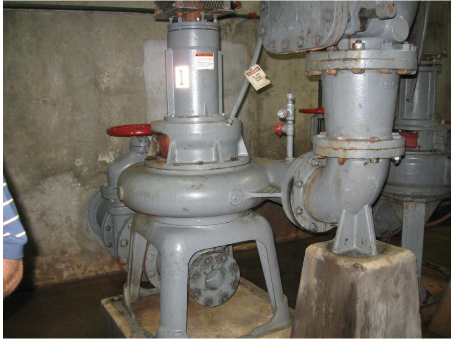
Figure 105-3. Chesapeake Blvd Pump No.1
