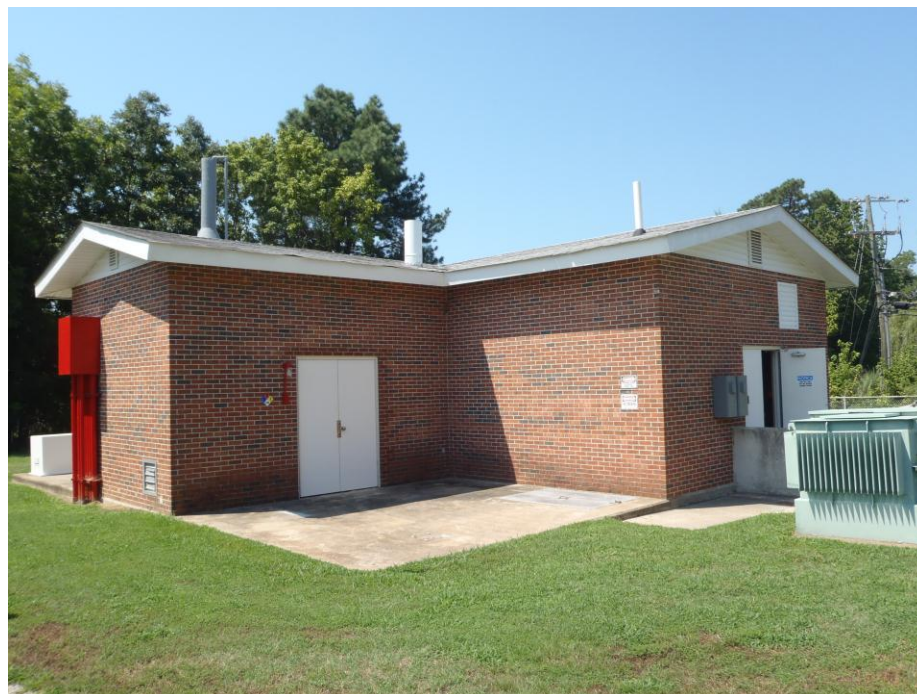
Figure 216-2. Lucas Creek Pump Station
