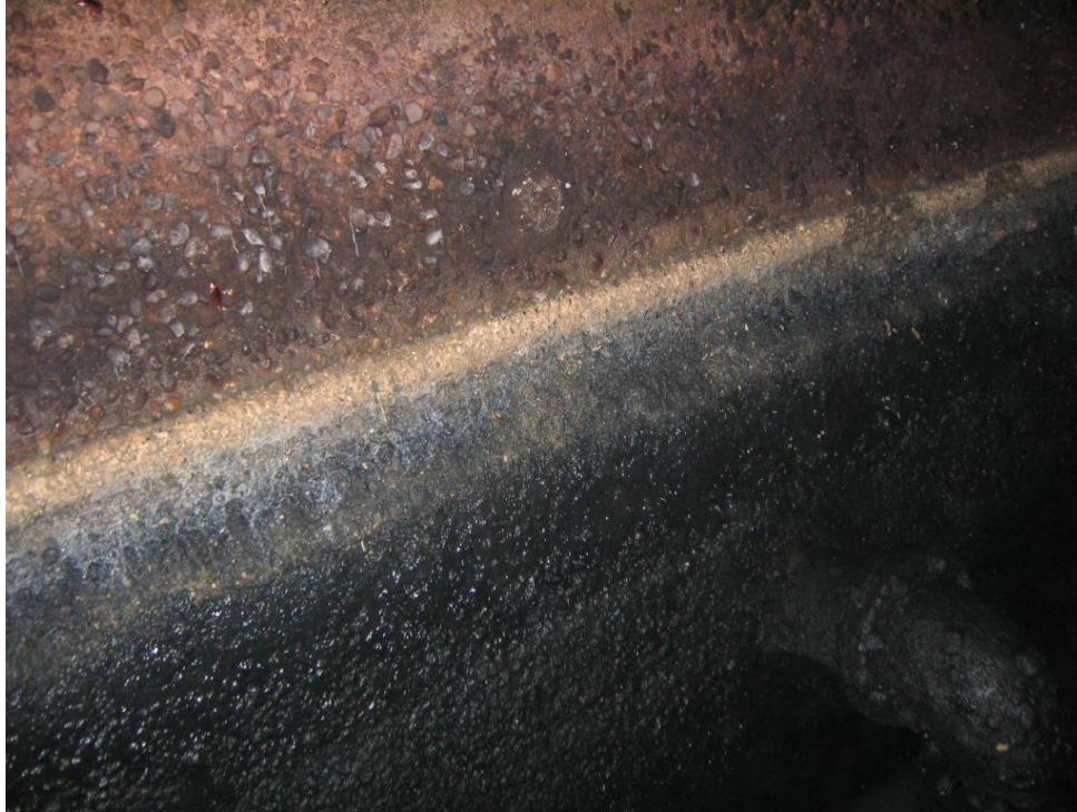
Figure 103-3. Bainbridge Blvd Wet Well
