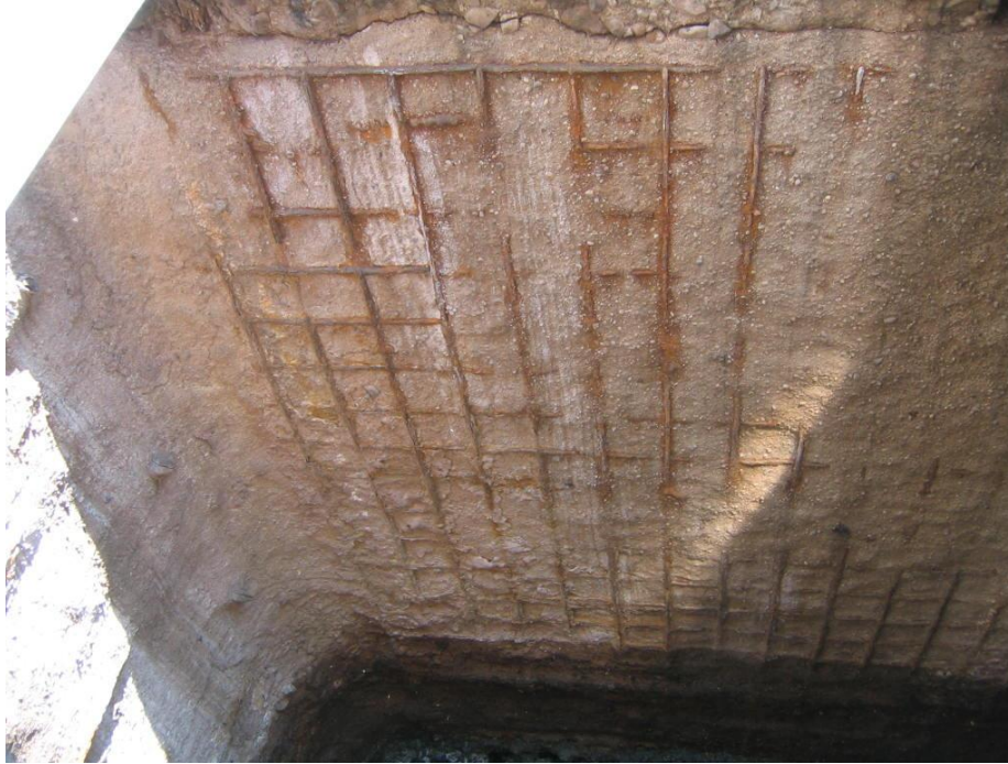
Figure 110-3. Wet well Photo No.1
