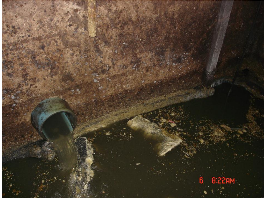
Figure 204-3. Bloxoms Corner Wet Well
