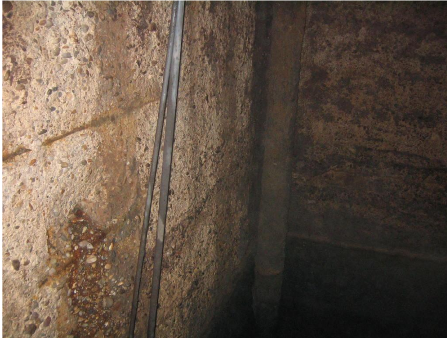
Figure 130-3. Virginia Beach Blvd Wet well
