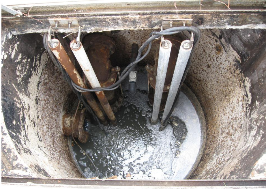
Figure 141-3. Hanover Ave Wet Well
