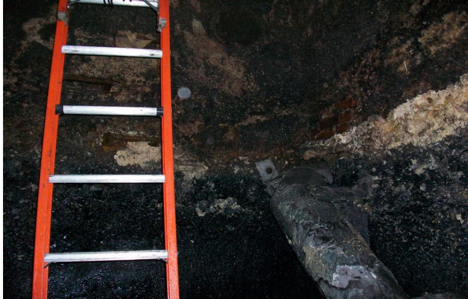
Figure 131-3. Washington District Wet Well
