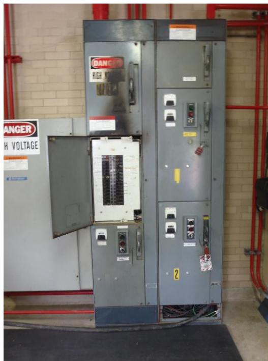
Figure 203-4. Bay Shore Lane MCC
