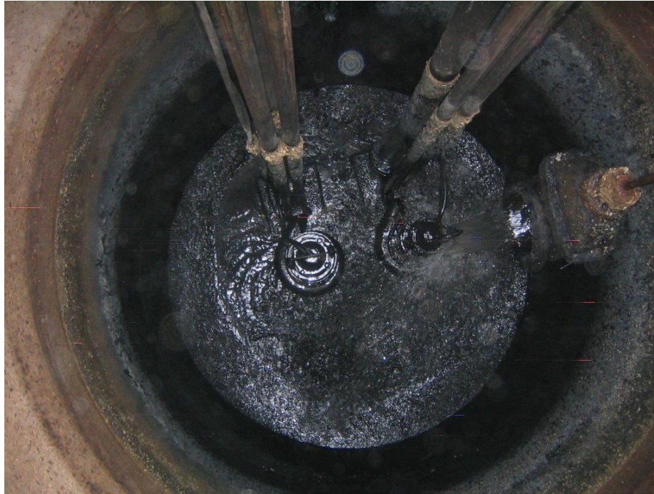
Figure 111-3. Granby St Wet Well
