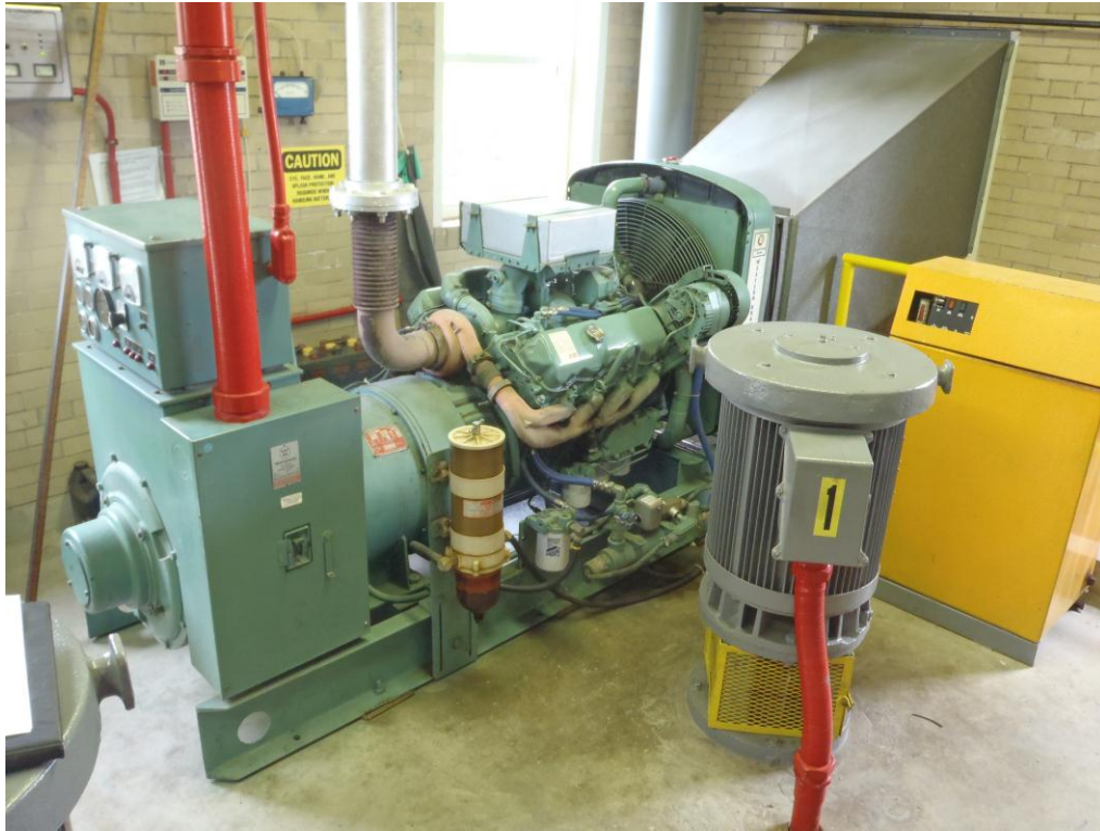
Figure 203-3. Bay Shore Lane Generator
