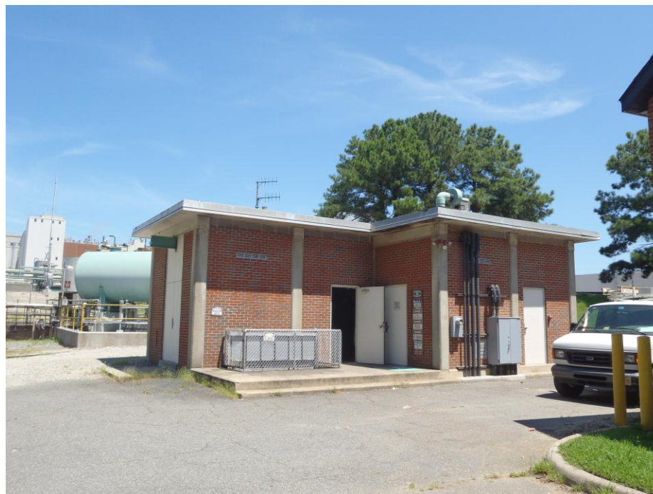
Figure 214-2. Kingsmill Pump Station
