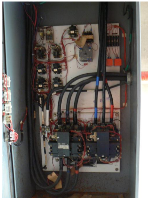
Figure 202-4. 33 rd St Transfer Switch
