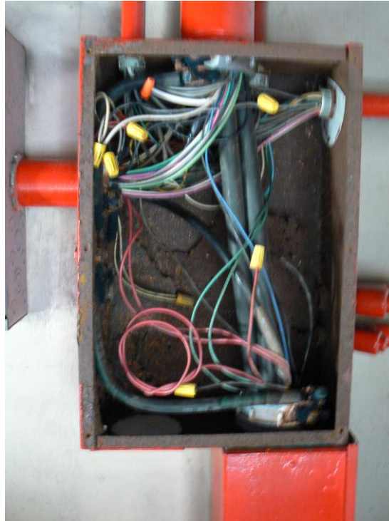
Figure 202-5. 33 rd St Junction Box
