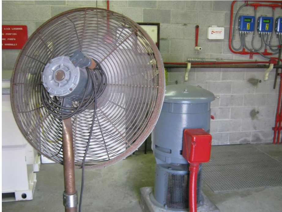
Figure 107-3. Motor No. 2 Cooling Fan
