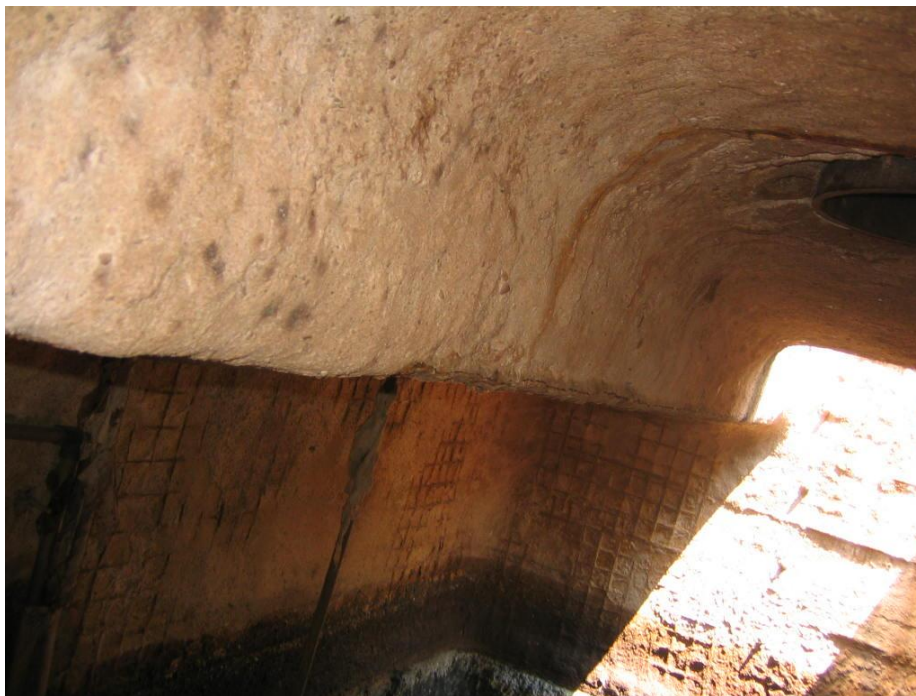
Figure 110-4. Wet well Photo No.2
