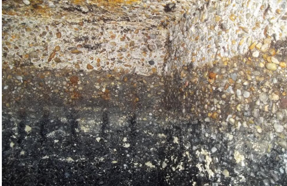
Figure 118-3. Typical Norview Ave Wet Well Concrete.
