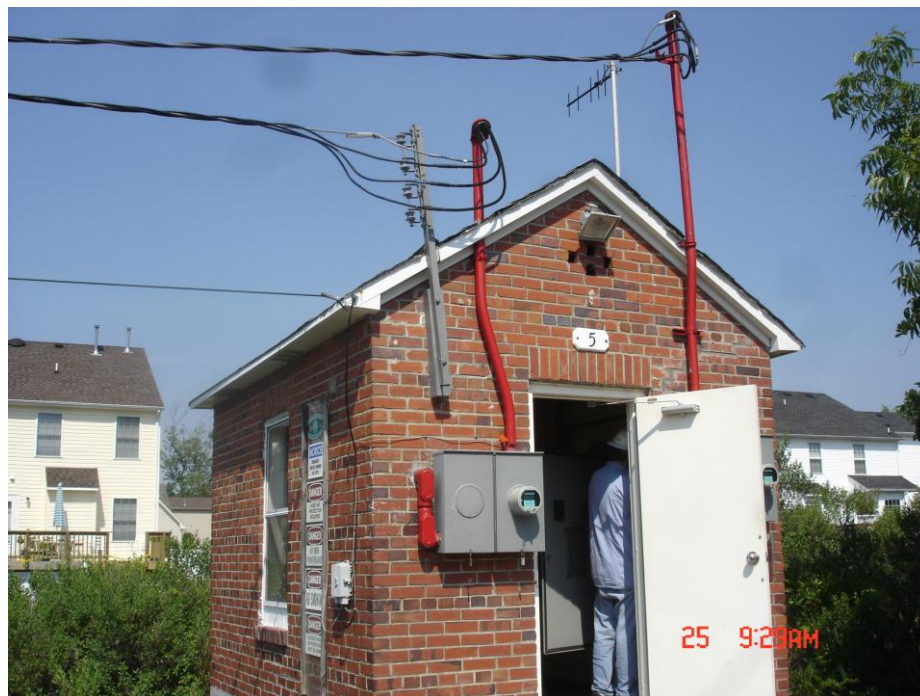
Figure 204-2. Bloxoms Corner Pump Station
